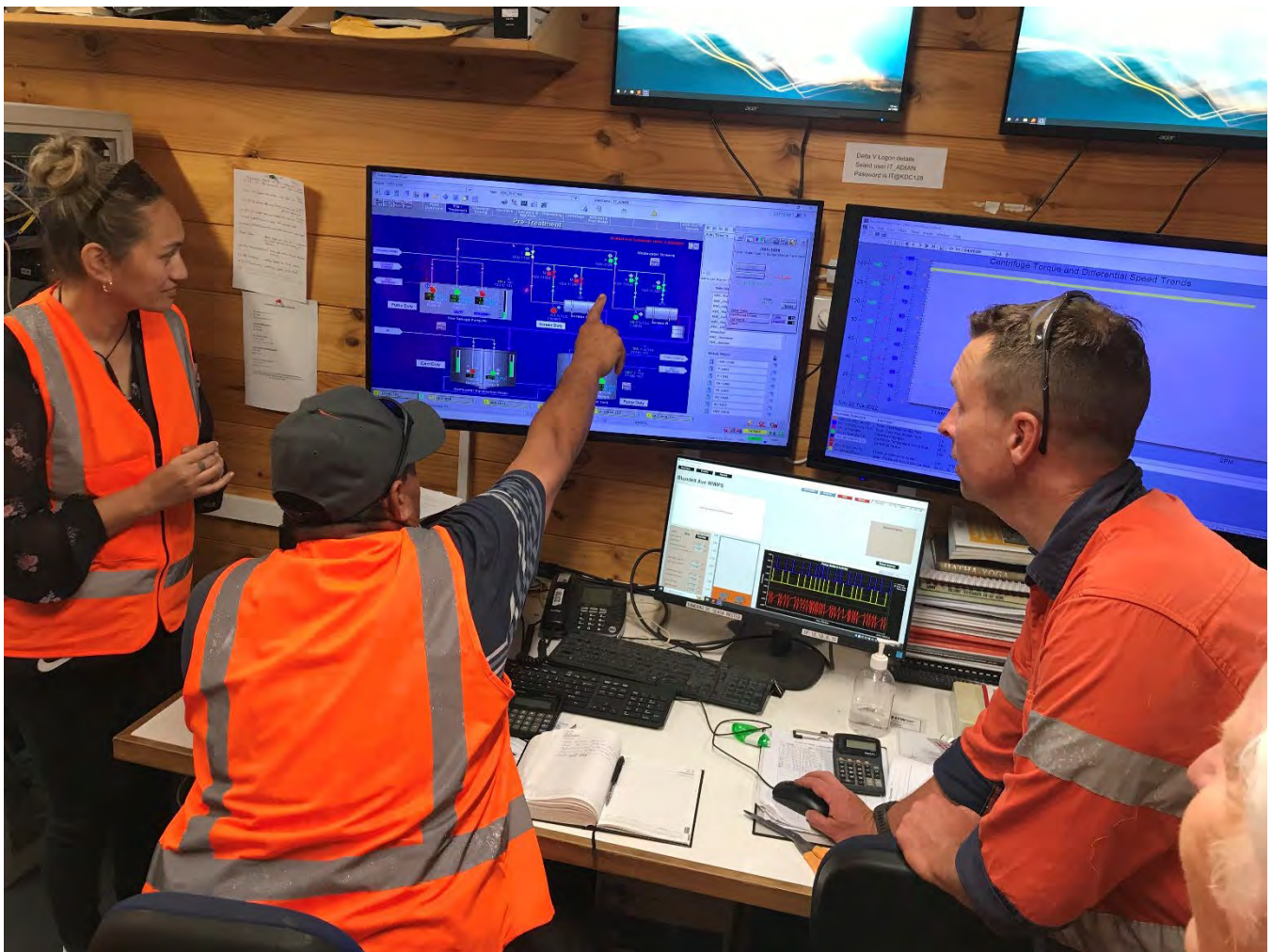
Mayor Faylene Tunui and Deputy Mayor view the new telemetry operations system installed at the Waste Water Treatment Plant control room with Three Waters Team Leader Glen Penny.
