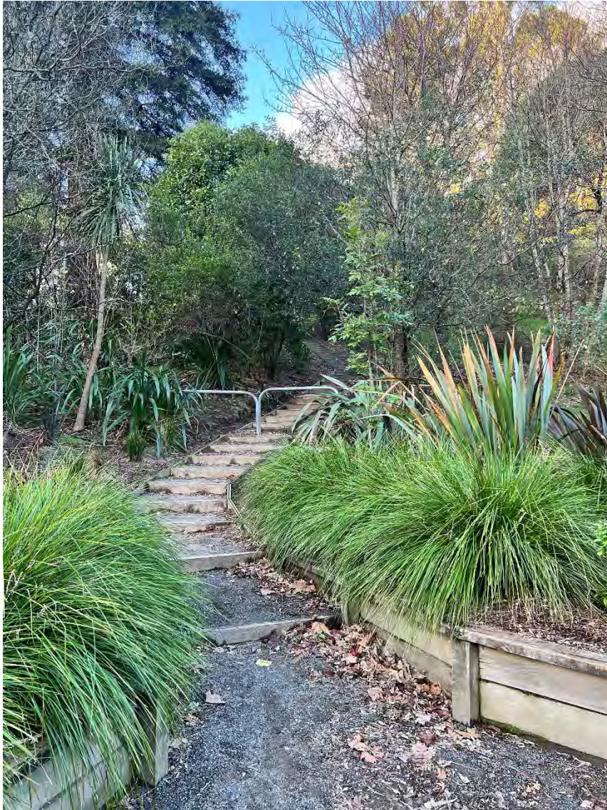
New stairs into Monika Lanham Reserve improved access after extreme weather damage
