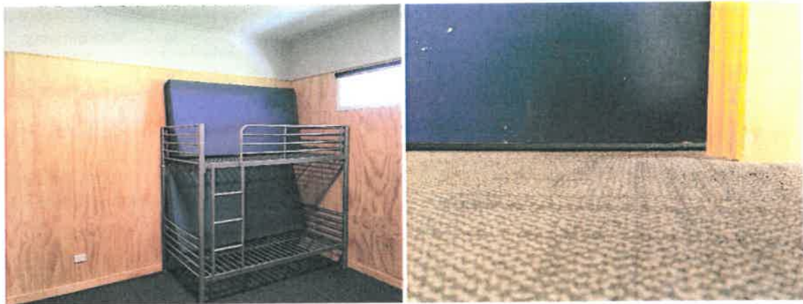
Figure 2: A photograph of the bunk room and the door undercut
